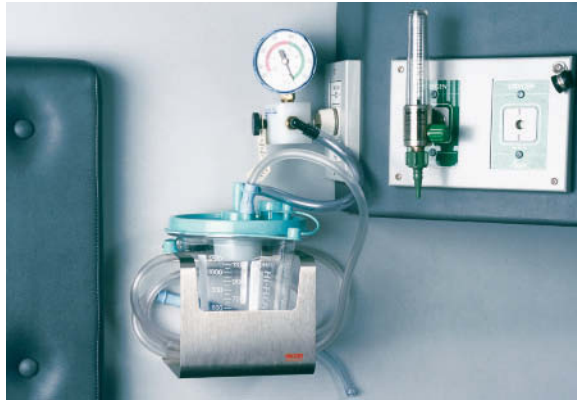
FIGURE 9-7 A mounted suction unit installed in the ambulance's patient compartment.
